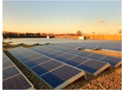
Sun Edison solar panels.
