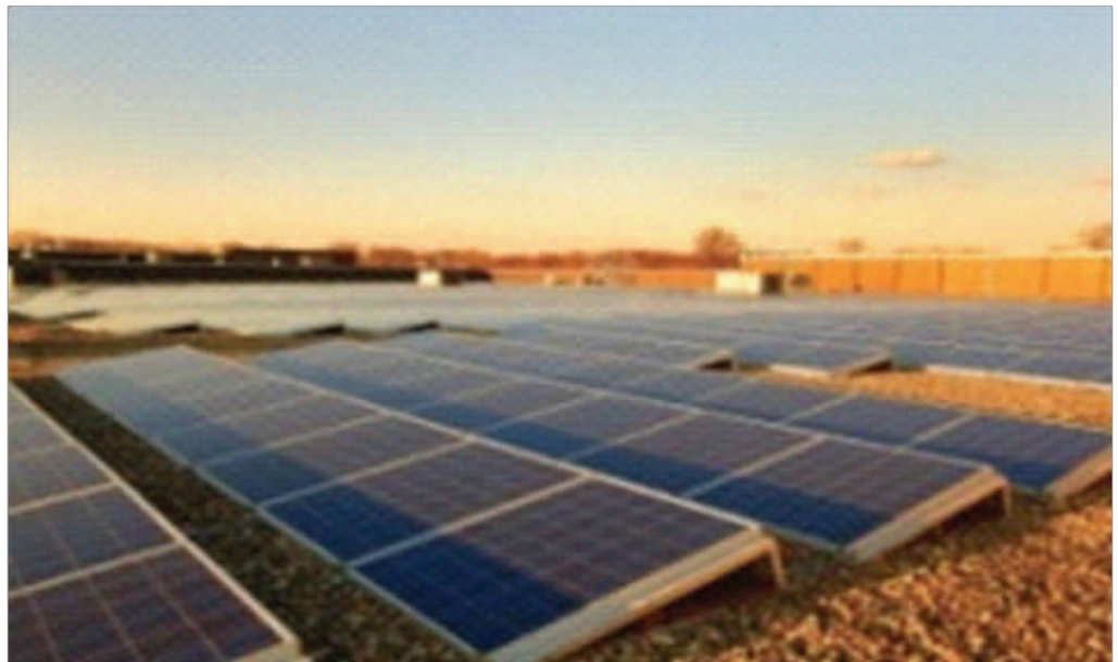
Sun Edison solar panels.
