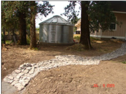
Rainwater Storage Tank at WISC
